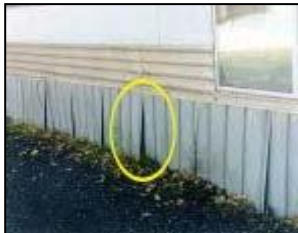
Fix gaps in trailer skirtings
