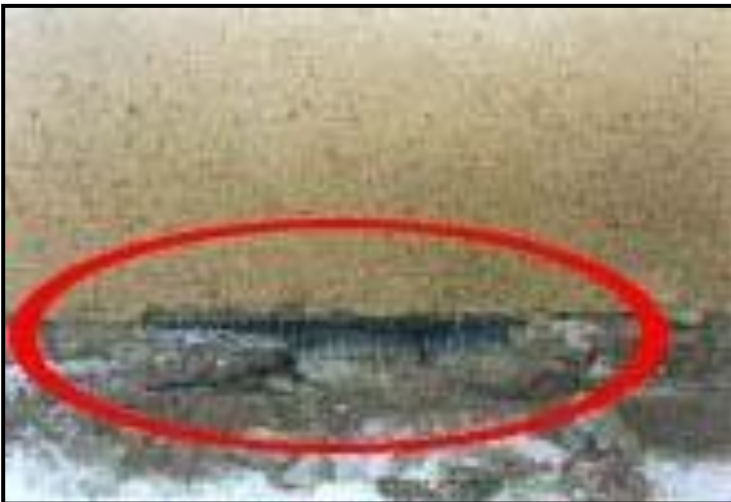
Fold lath metal and place in holes in the foundation of houses
